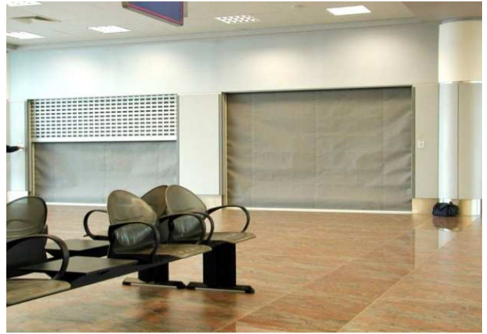
Fire shutters - Airport Václav Havel - Prague
