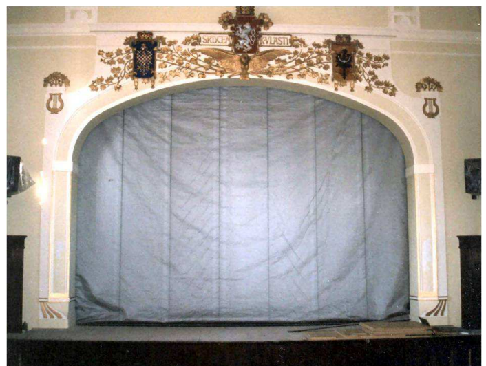
Fire shutter in theater
