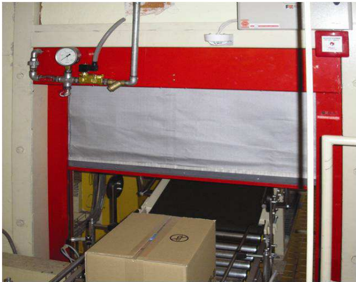
Fire shutter installed on conveyor belt
