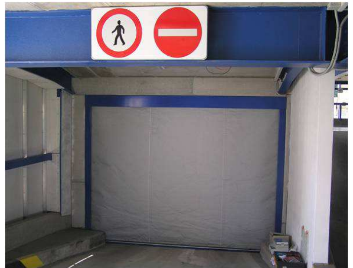
Fire shutter in garage
