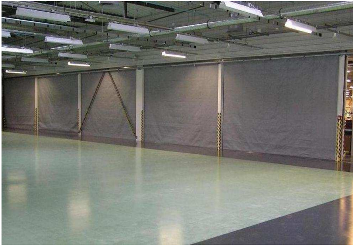
Fire shutters in manufacture hall
